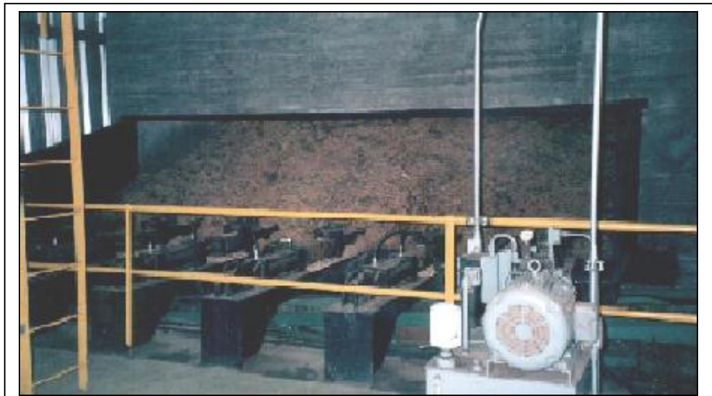
Figure 2 typical hydraulic cylinders and pump arrangement.
