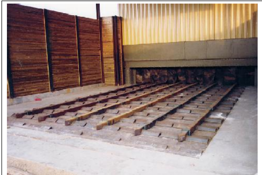
Figure 1 A typical reciprocating floor unit. Notice the main assembly is mounted on a single steel plate rather than to the concrete
