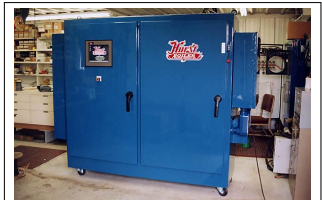
Figure 13 HBC's Boiler Fireman Control Cabinet
